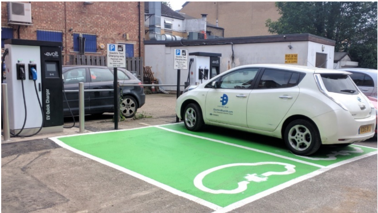
A charging point for taxis in Cambridge
